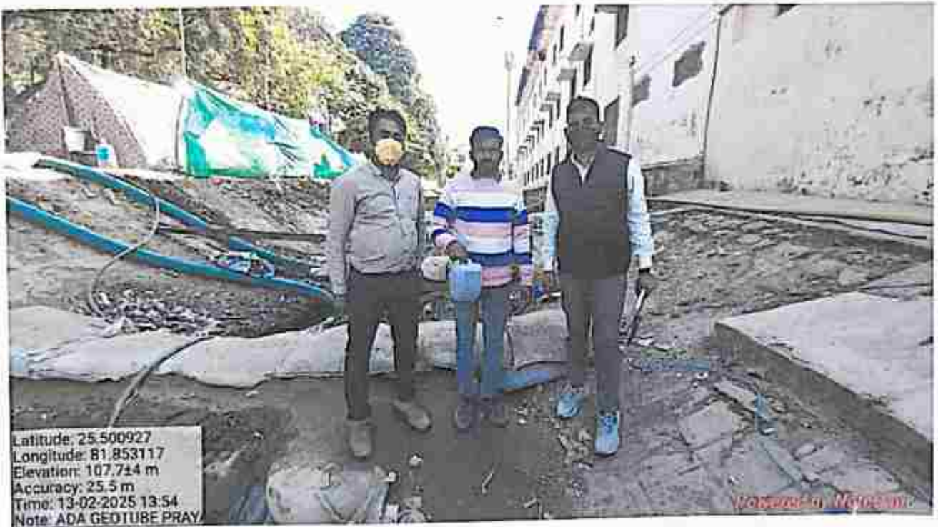
ADA Geotube, Prayagraj
