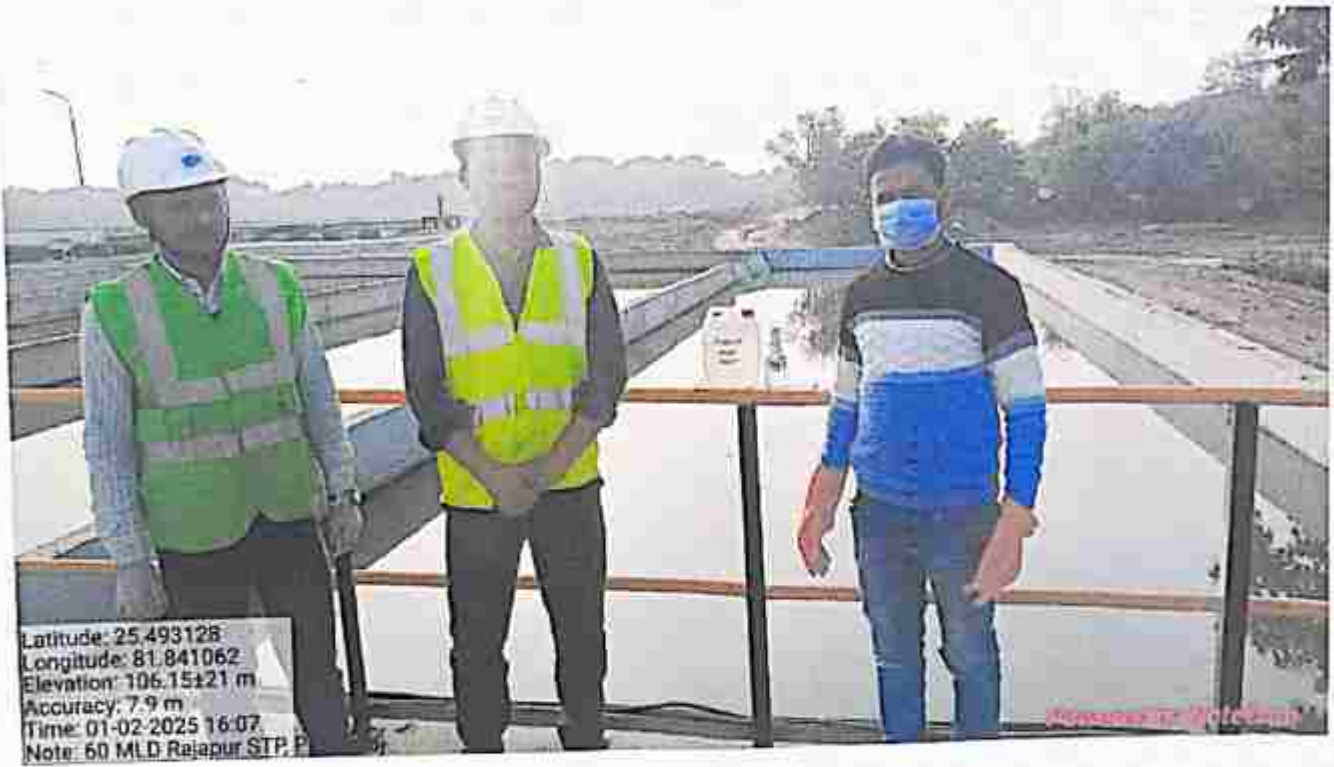
60 MLD Rajapur STP, Prayagraj
